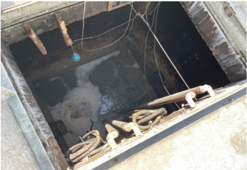
Photo 11: View inside wet well at station; no significant buildup of grease, grit, or major corrosion observed.
