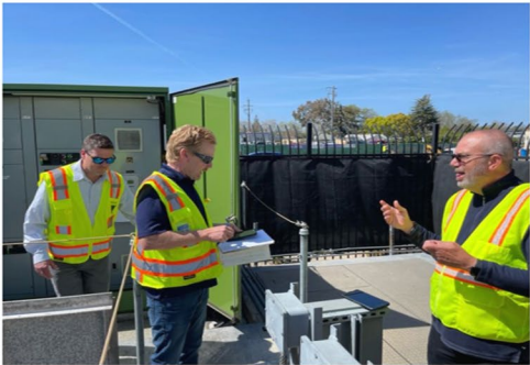
Photo 12: Inspection with operations staff on station operations, maintenance, bypassing, wet well holding time, and other details.
